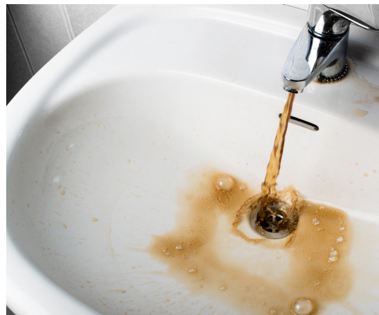
Discolored tap water due to pipe corrosion.
